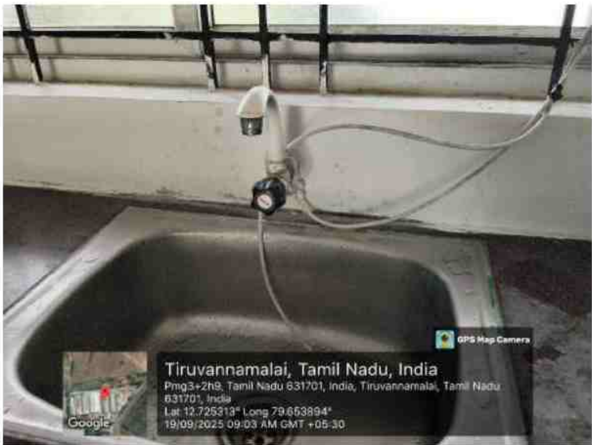
Photograph of low flow type aerator in pipe
